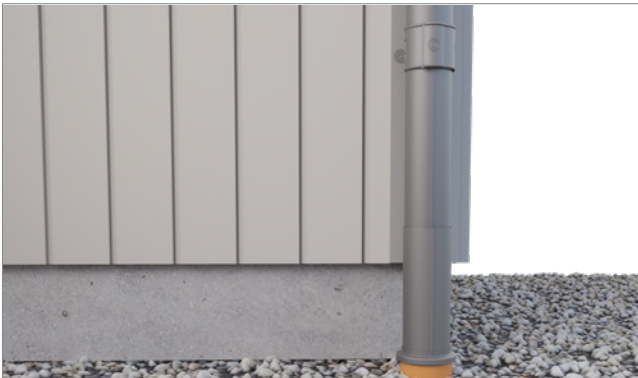
A BUTK drain shoe is connected to an unenclosed ground drain pipe.
